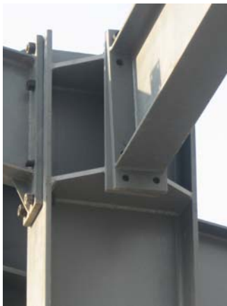
End Plates no coinciden
